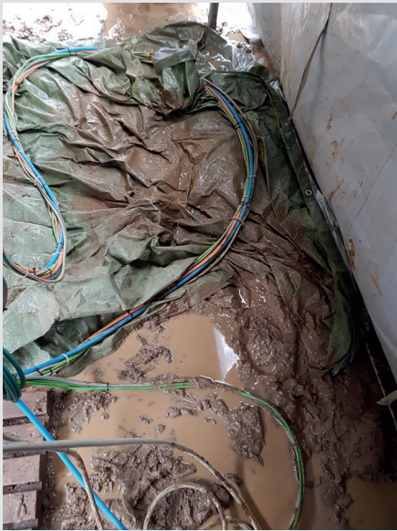
Figure 10: Fiber optic hose package in soggy soil
