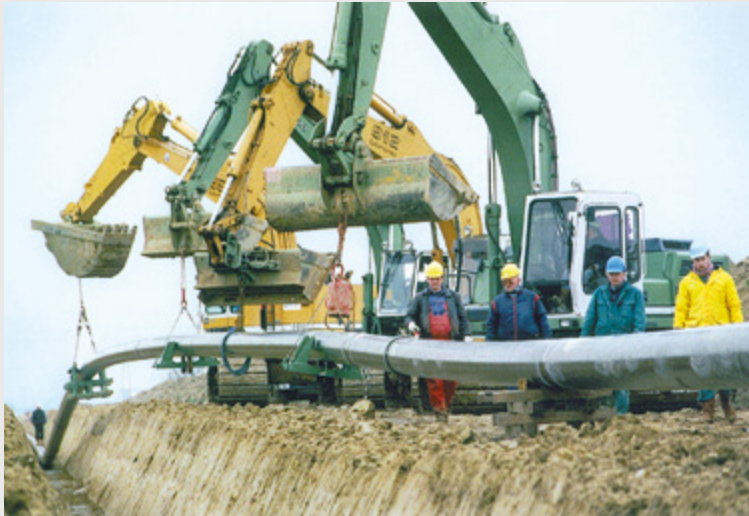
Figure 3: Bend radii in a welded pipe string being lowered into the trench
